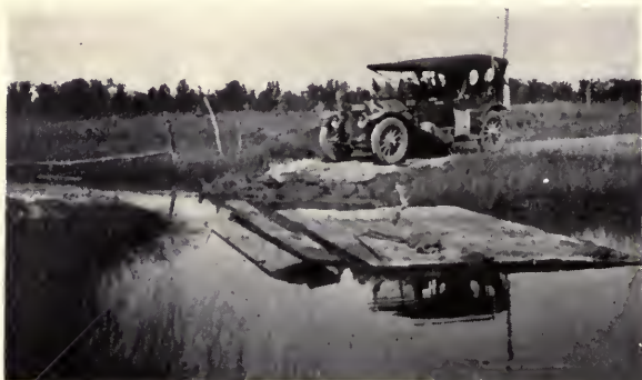
This situation, encountered in Montana, necessitated the taking apart and reconstructing the bridge. Laborious and slow but counted as all in the day's work
